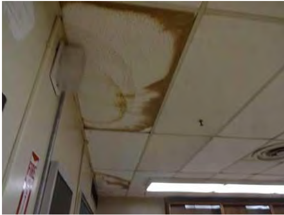
6 th Floor Roof Leaks
