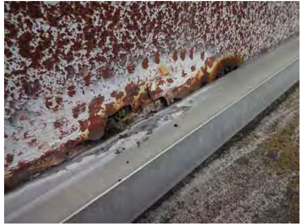
Damaged Wall Panel on West Wing
