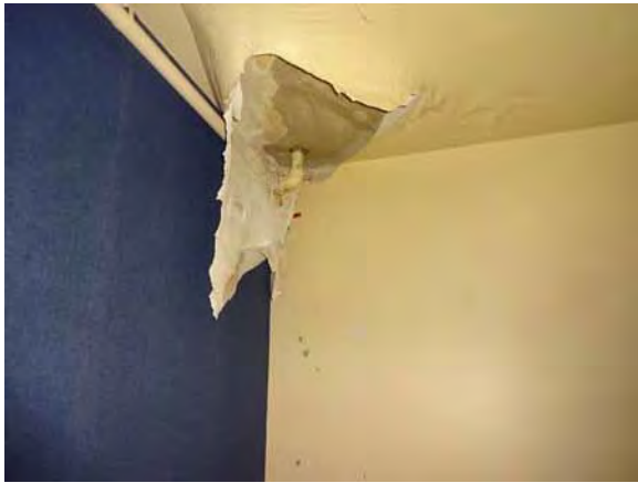
Roof Leak in Auditorium
