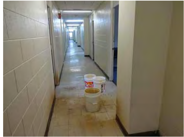
Third Floor Corridor (Buckets for Roof Leaks)
