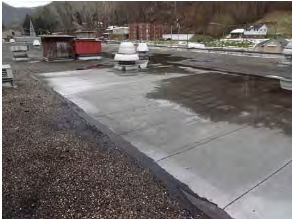
Old Roof Patch
