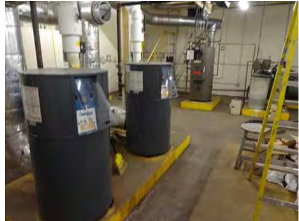
Mechanical Room in Lower Level
