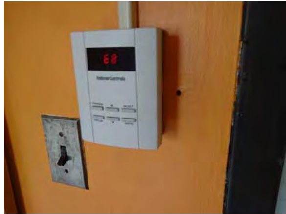
Local Thermostats Control Units
