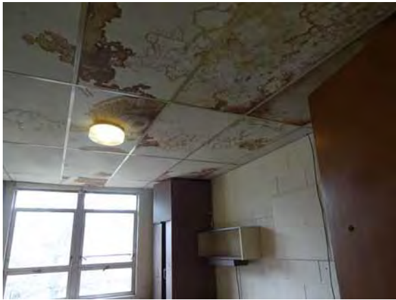
Evidence of Roof Leaks
